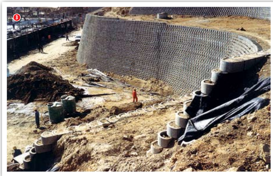
1 This CRB retaining wall at Montecasino in Fourways, Johannesburg, was completed within four months
